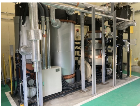
[Biomass boiler at the Ibaraki Plant]
