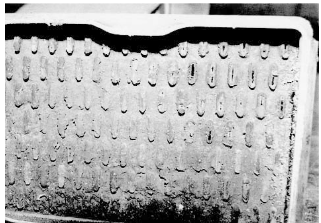
Photo 2 Radiator clogged with scale (section of radiator top tank side)
