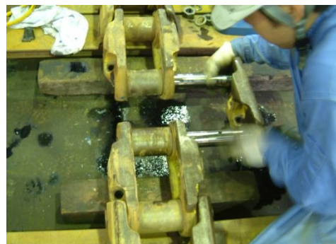
(3) The outer link and pin on the opposite side are simultaneously removed.
