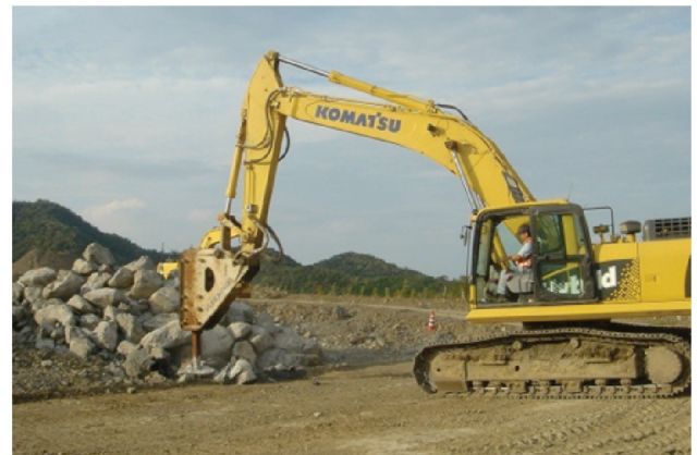
Fig. 16 Breaker installed (From internal document)
